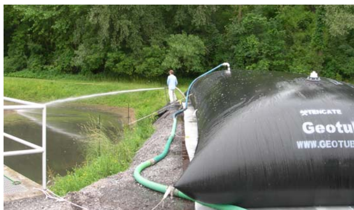
The lagoon residuals were homogenized by high-pressure spraying. The Geotube® container is being filled and is dewatering properly.
