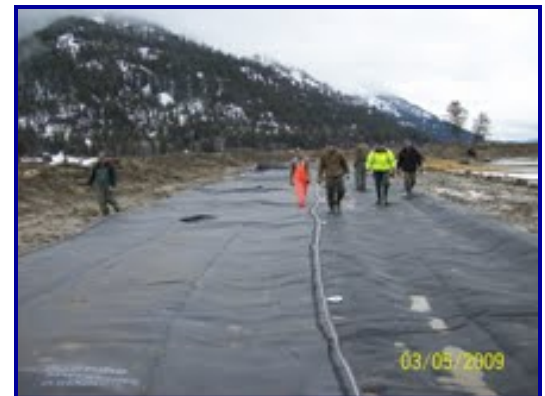
(Right) Geotube® unit laid out on scour apron ready to start filling.
