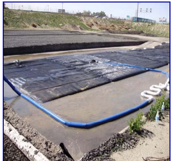
The blue soft hose transfers the chemically treated biosolids to the mixing manifold and Geotube® container.
