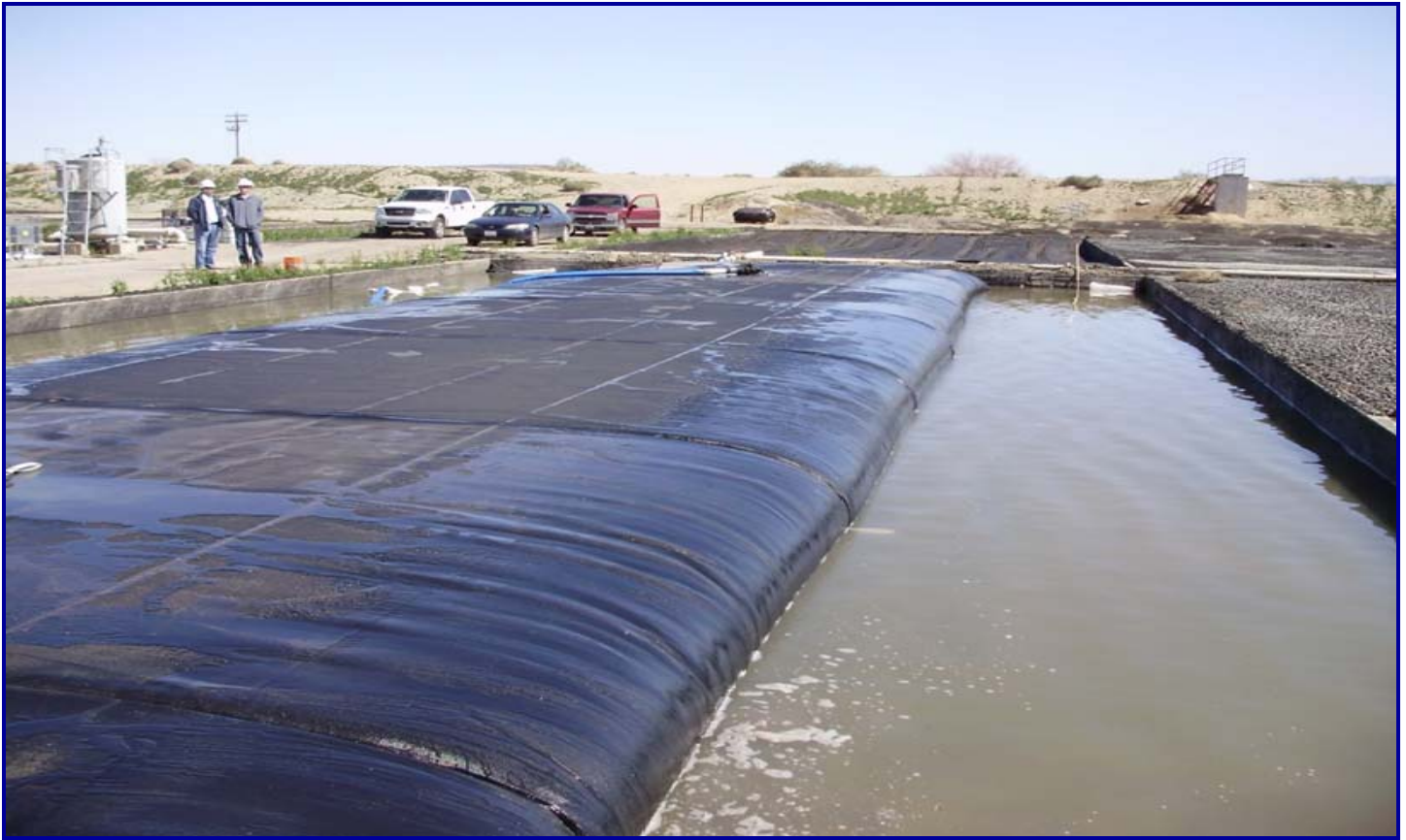
A 45' circumference by 100' long Geotube® container is dewatering in the drying bed.
