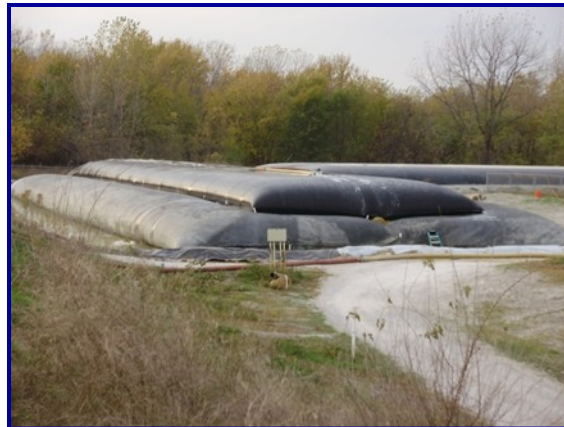
The Geotube® container is stacked to make the most of the space available at this site.
