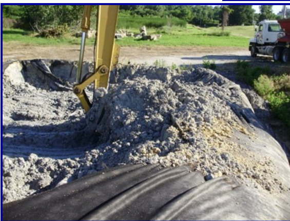
The residual in the Geotube® containers is being hauled away with dry wt solids ranging from 25 to 33%.
