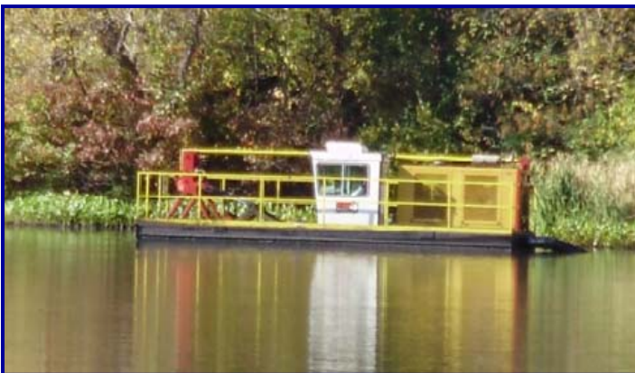
Dredge pumped at approximately 2,000-gpm with the assistance of an in-line booster pump.
