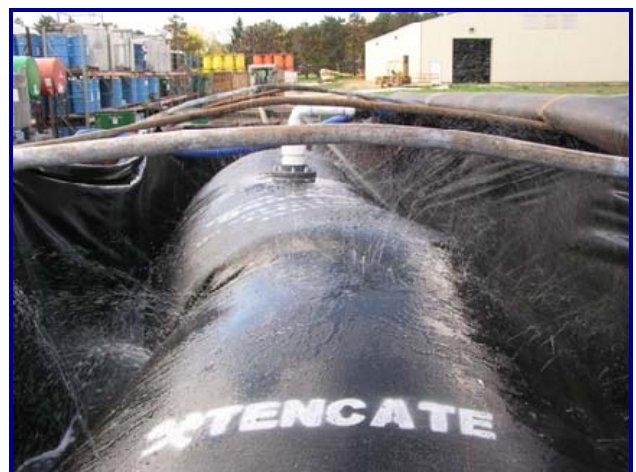
The Geotube® container filled to capacity and dewatering with tiny sprayers exiting the tube.
