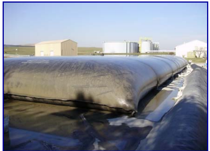
The Geotube® container is continuing to dewater. It was filled in November and will be excavated in the upcoming summer.
