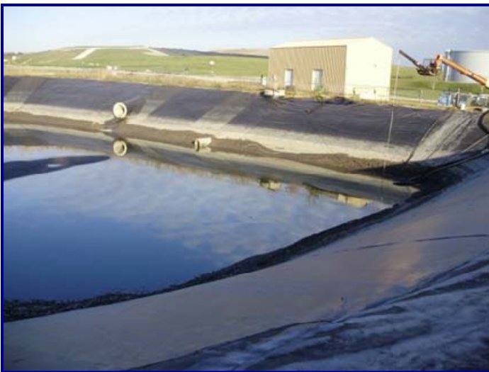
The pond had approximately 3' of mud in it when we arrived. One half of the solids were removed in the week long dewatering process.
