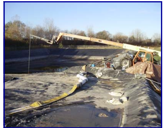
The telescoping forklift is holding the hydraulic pump in the settling pond and the 6" hose coming from that pump is connected to the white mixing manifold in which the polymer is injected.
