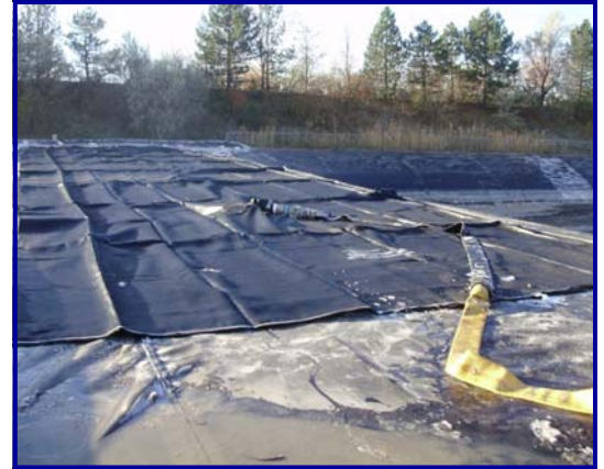
This Geotube® container was placed on the containment pad at the end of the holding pond and the filtrate drained back into the pond.
