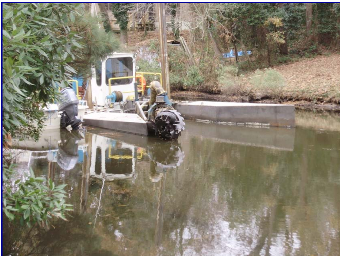
This hydraulic dredge dug through the canals and out into the sound sending the mud and sand to the lagoons at 2200 to 3000 GPM in a 10” pipeline.
