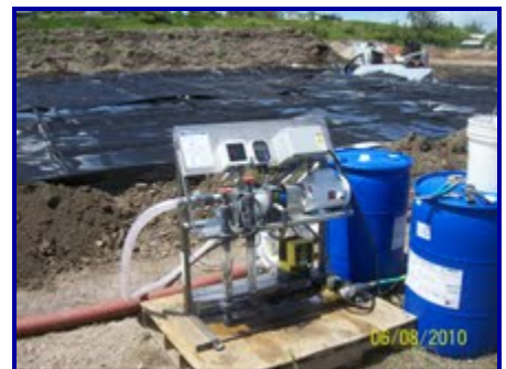
Using WaterSolve's WSLP 2400 unit for chemical addition and Solve 137.
