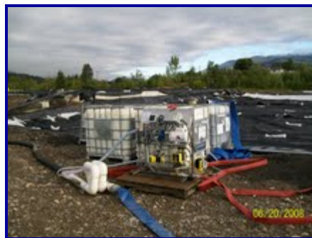
WaterSolve's chemical conditioning unit (WSLP2400), totes of Solve 152
