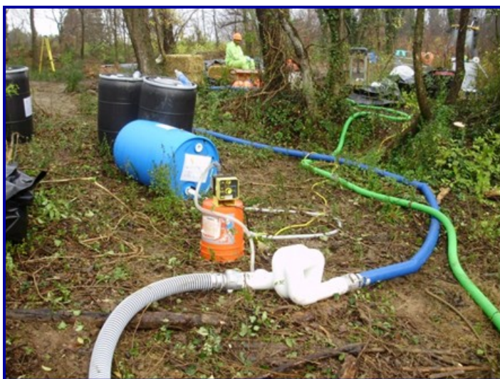
The coagulant Solve 426 is injected into the 3" mixing manifold .
