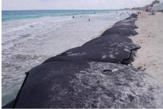
A total of 1.24 miles of Geotube® units were used for emergency protection and restoration.
