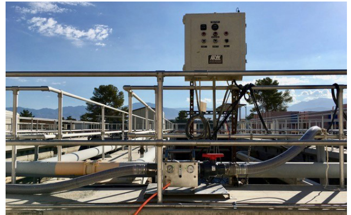
Aerobic digestion tanks at the city's municipal wastewater treatment plant
