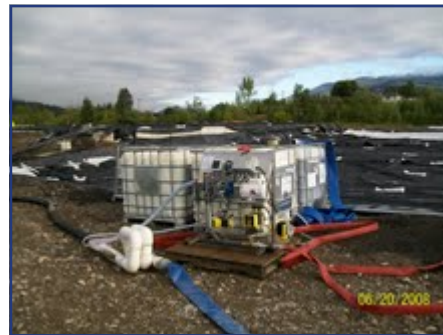
The chemical conditioning unit and totes of Solve 152 and Solve 426.
