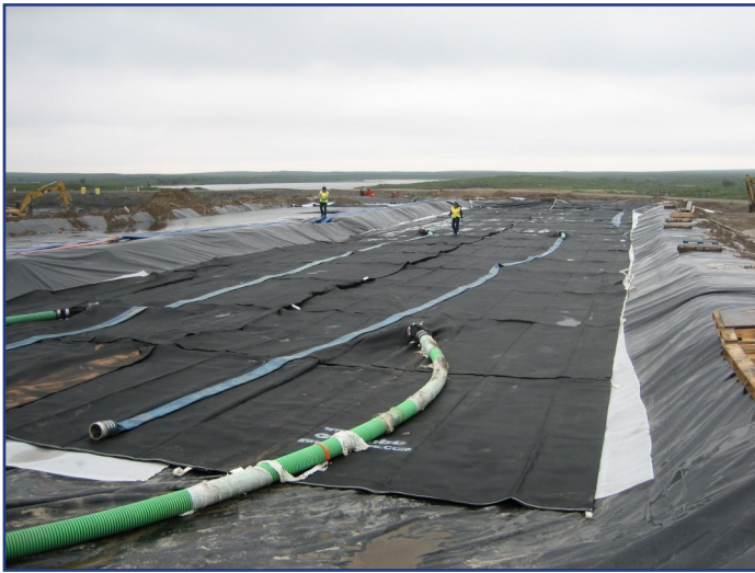
Two 45' circumference by 200' length Geotube® containers were placed for each treatment train and connected with hoses.
